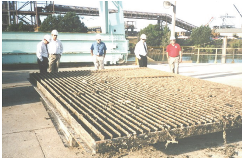
Intake Trash Bars
