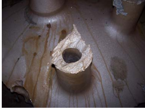
Safety nozzle after flange removal
