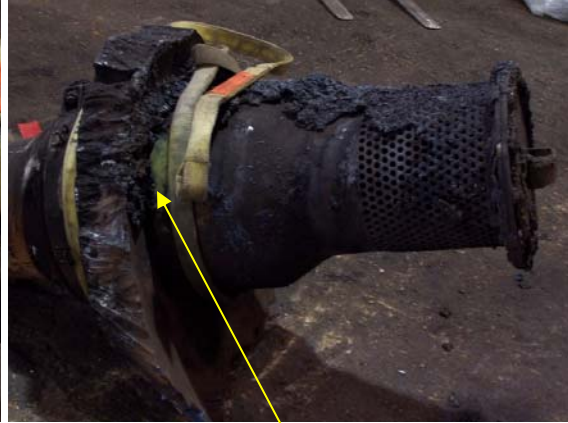
Internal portion of Surge nozzle
