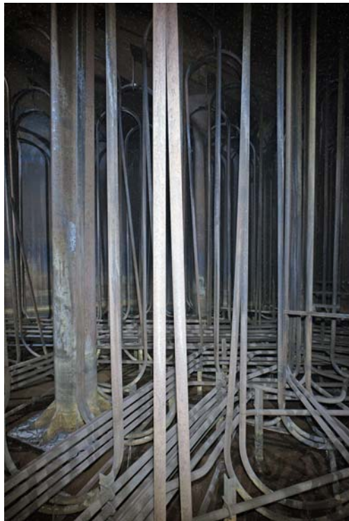
Figure 2.1-33: Typical Type I Waste Tank Cooling Coil Obstacles
