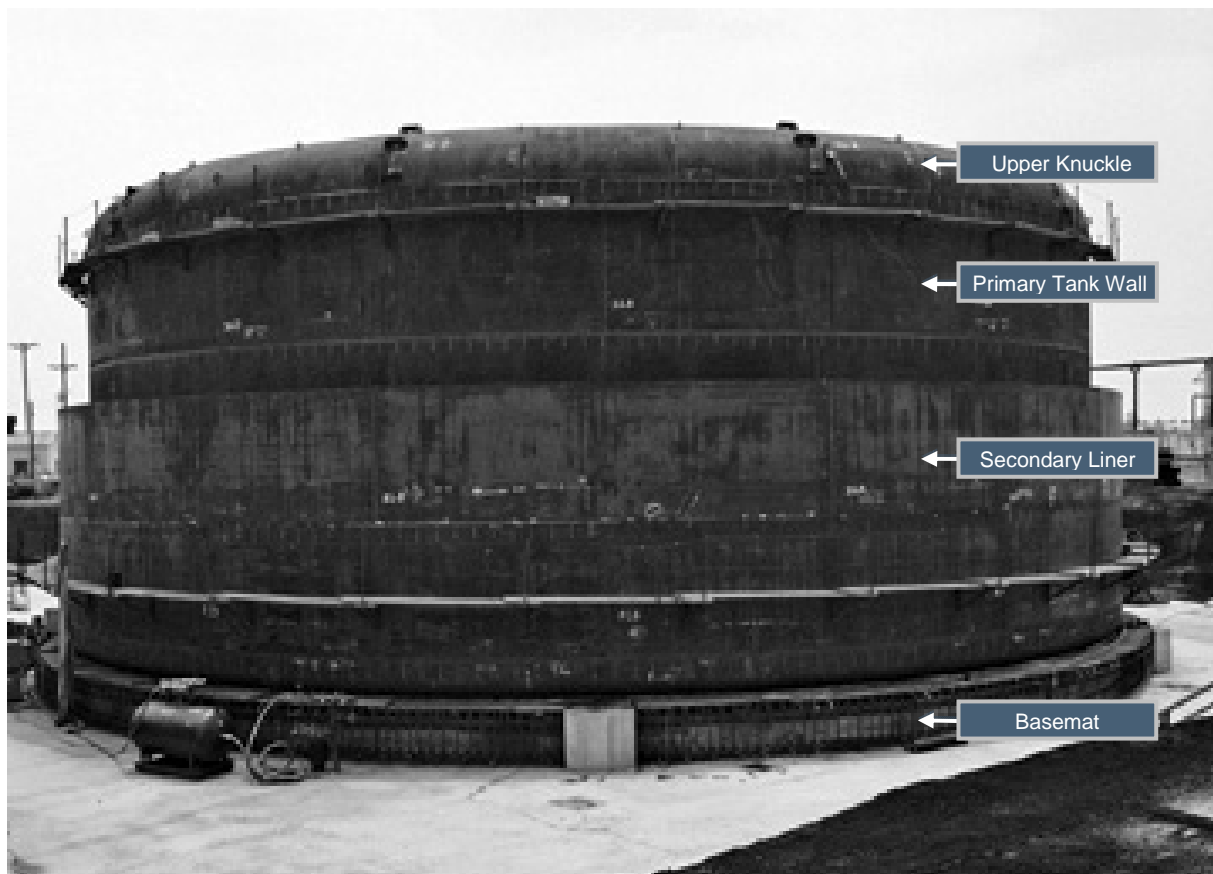
Figure 2.1-38: Typical Type IIIA Waste Tank Primary Tank and Secondary Liner - Late Construction (Vault Wall Not Constructed)
