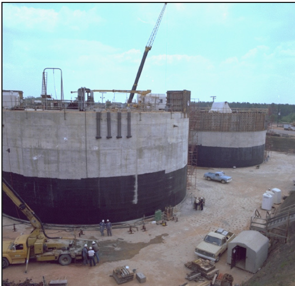
Tanks under construction. Note tank size relative to construction workers. Later, dirt is backfilled around the tanks to provide shielding.
