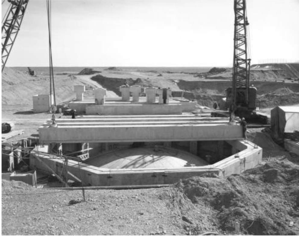
Figure 1-3. Vault and dome of Tank WM-185 showing the concrete beams and concrete risers on top.
