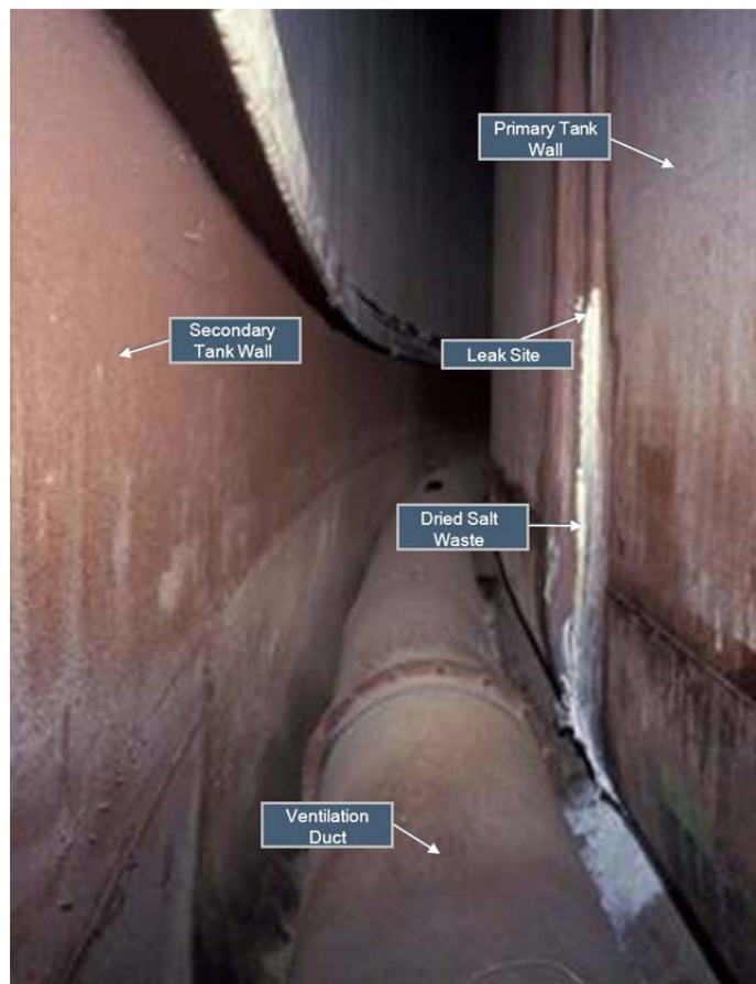
Figure 2.3-7: Waste Deposits on Exterior Primary Tank Wall Before Cleaning (Tank 5)
