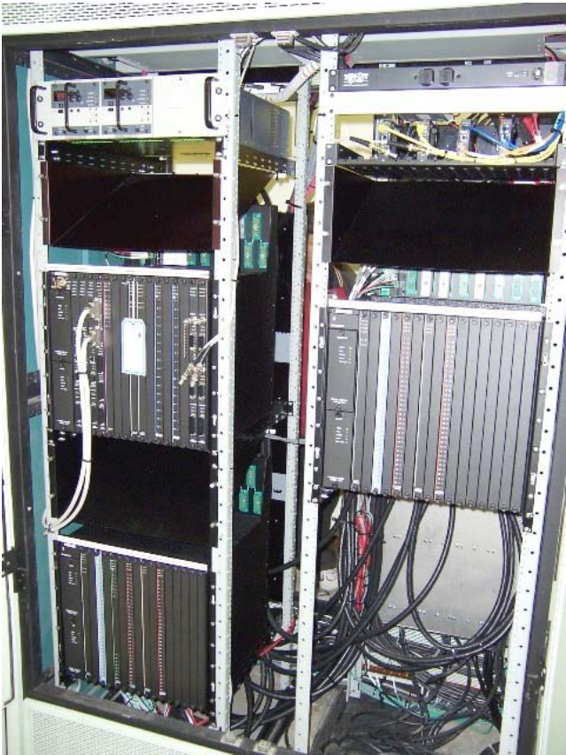
Figure 1-53 New Equipment Mounted in Cabinets
