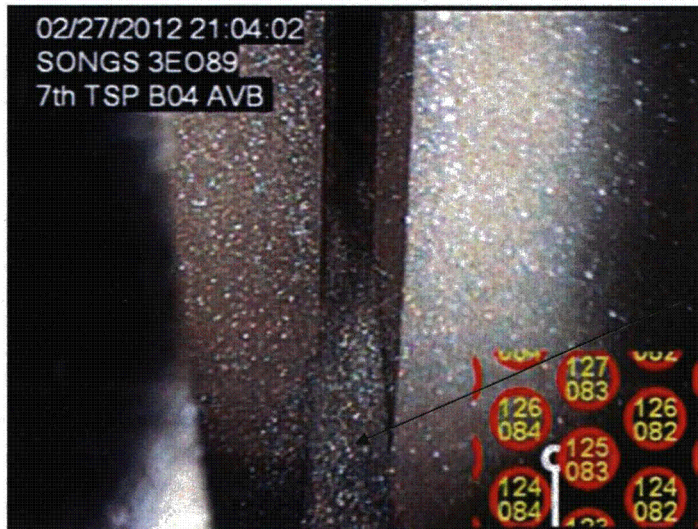
Photo-6 Tube Bundle Visual Inspection Image [Unit-3A]
