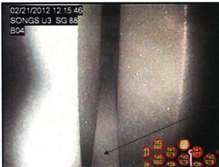
Photo-7 Visual Inspection Image of Outermost Tube Region [Unit-3B]
