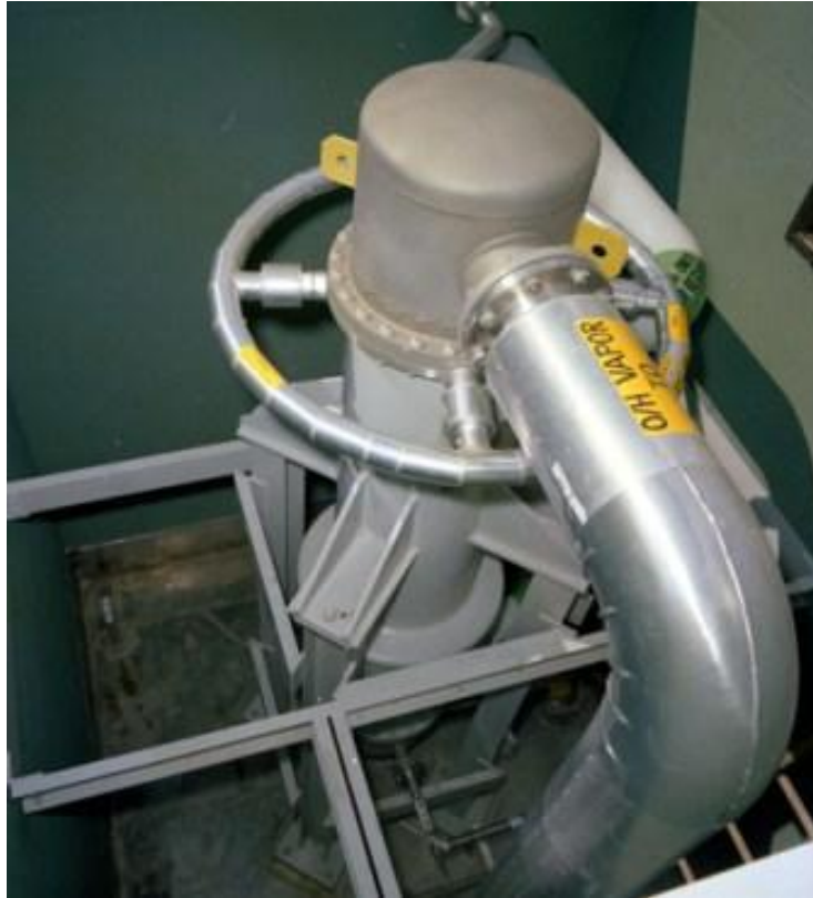
Figure 3.2-71: 242-25H Evaporator Overheads System Condenser
