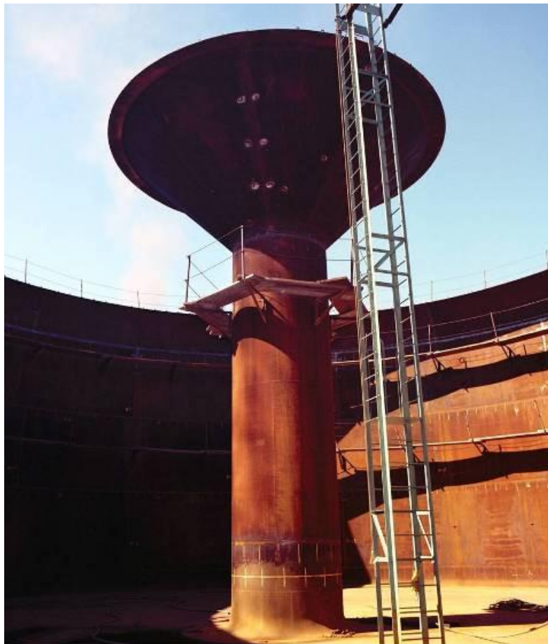
Figure 3.2-35: Typical Center Column Roof Support in a Type III and IIIA Tanks
