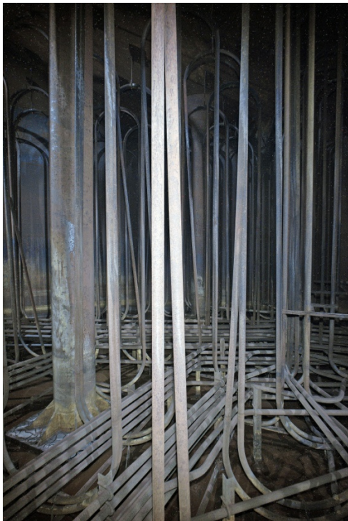
Figure 2.1-33: Typical Type I Tank Cooling Coil Obstacles
