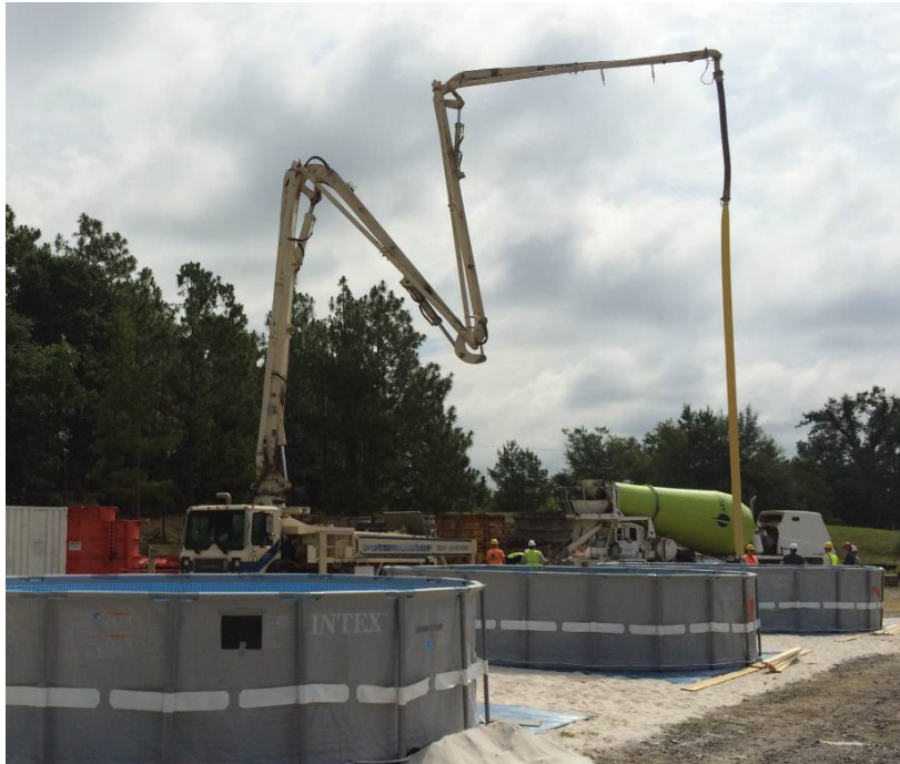
Figure 1. Grout Drop Test Molds with Boom Pumper Truck and Tremie (Photograph Adapted from RPT-5539-EG-0016).
