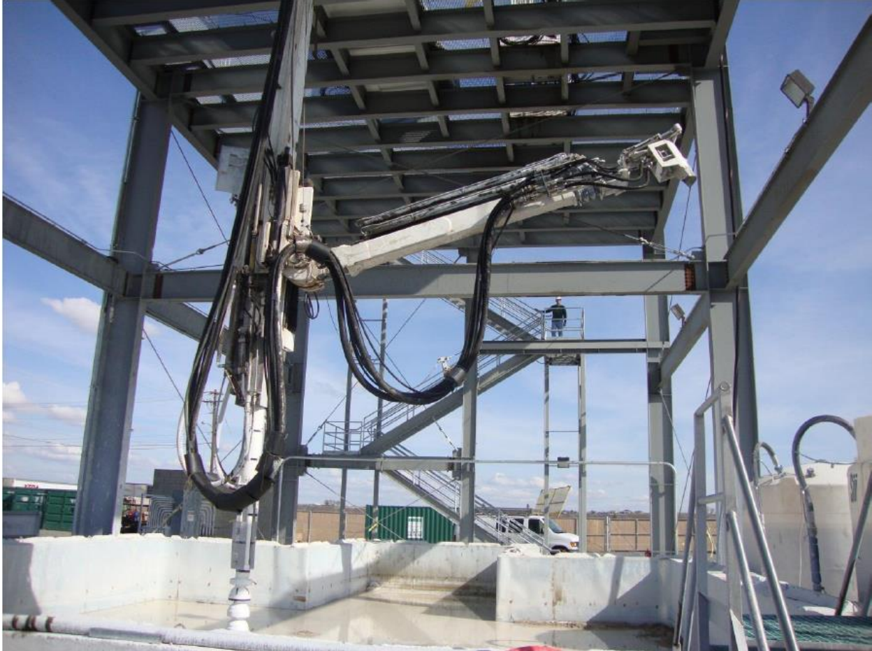
3 Figure 2-22. Sluice-Mode Mobile Arm Retrieval System In-Tank Components.
