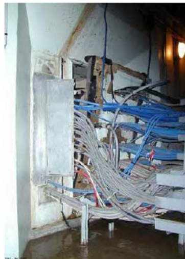
Failure of Cable opening
