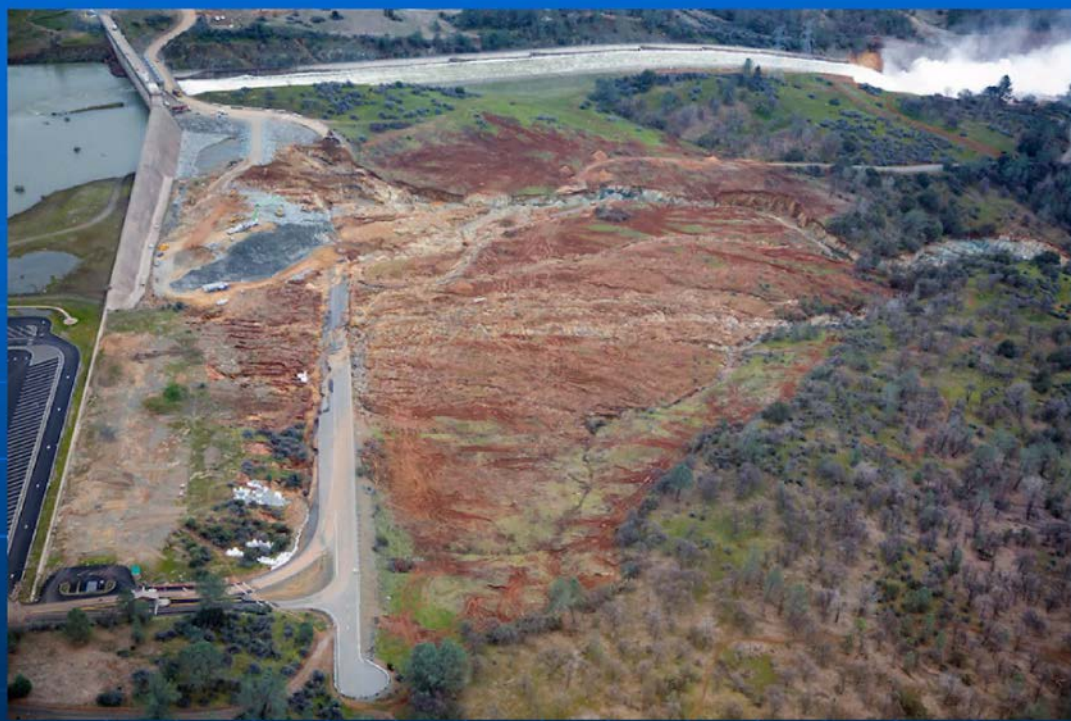
Emergency spillway erosion as the result of 12,600 cfs discharge
