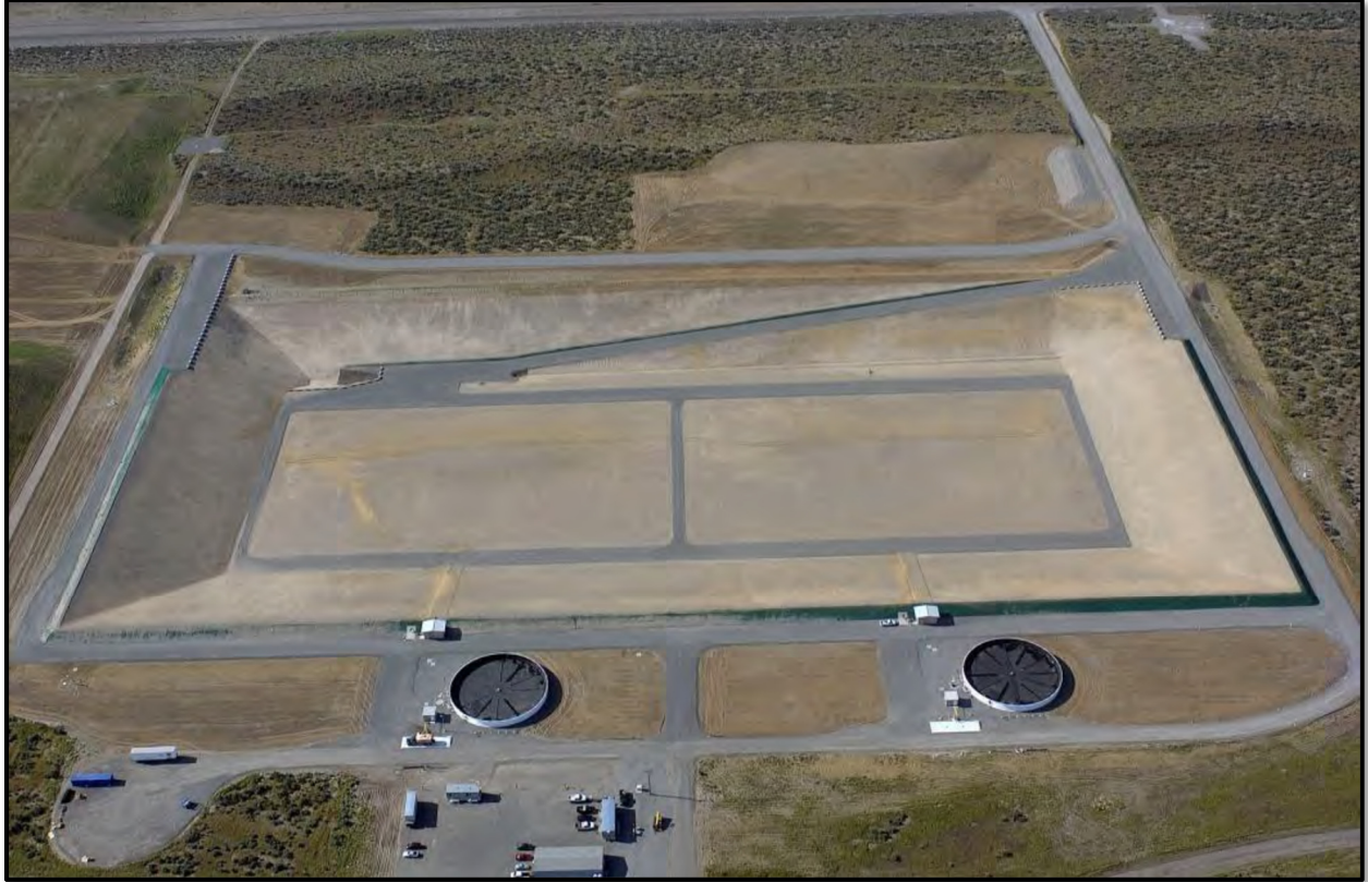
Figure 2-26. Integrated Disposal Facility Cells 1 and 2.
