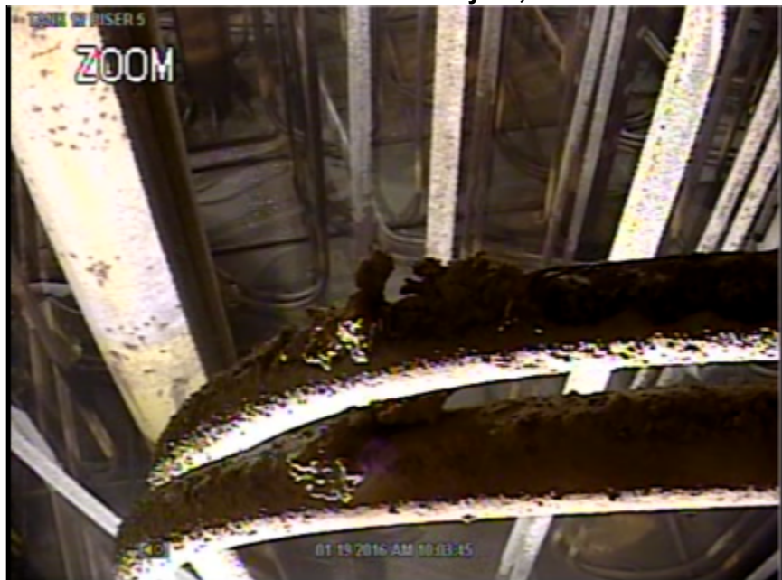
Figure 2. Residual WIR on cooling coils within the Tank 12H Primary. Date of Video: January 19, 2016.
