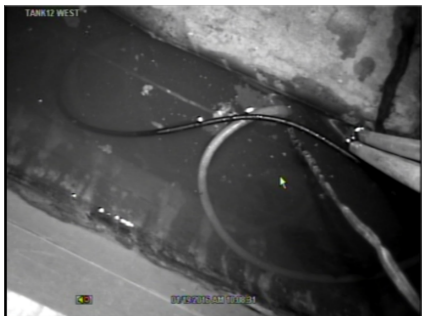
Figure 4. Groundwater In-Leakage in the Annulus, as viewed from the West Riser. Date of Video: January 19, 2016.
