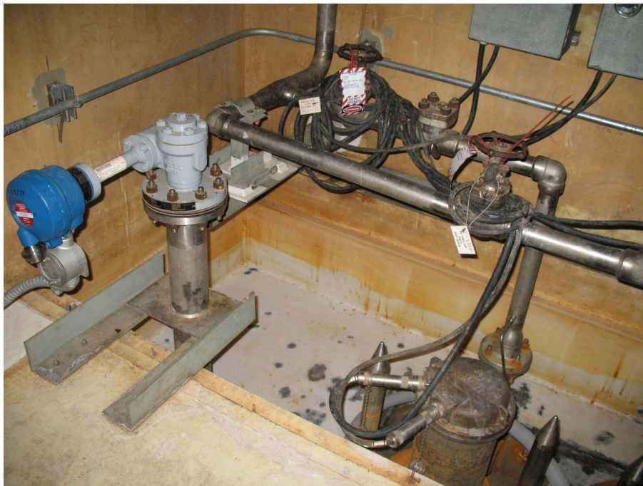
Figure 3-11 Sump well and recirculation system. (Generic photo.)
