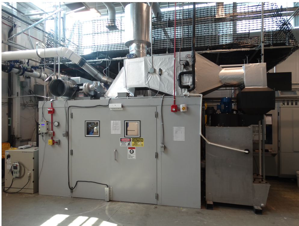
Figure 1-2 Helium recovery system installation (courtesy of ARL).
