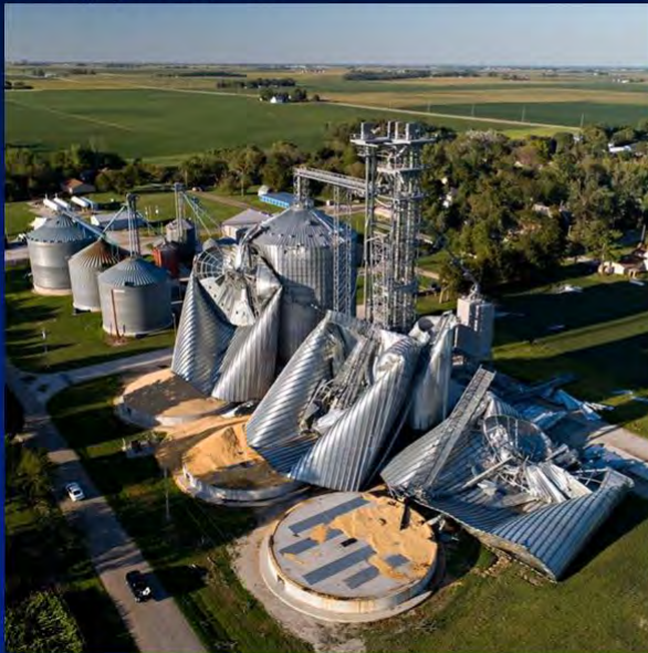
Storm damage from the derecho – State of Iowa, 10 August 2020
