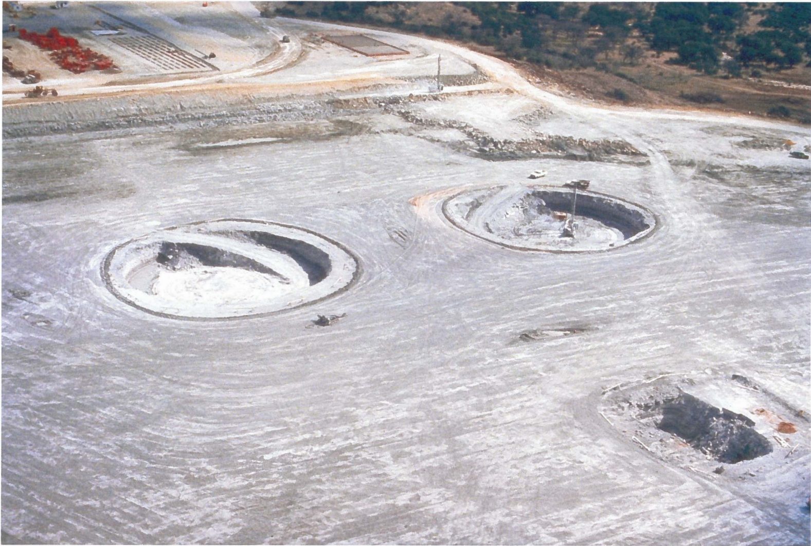
Figure 3.8-6 Construction Photograph of the CPNPP Site After Tree Removal, Mechanical Leveling, and Initial Excavation
