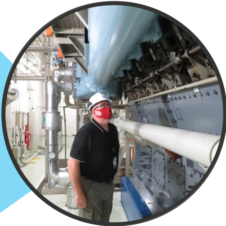
Senior Resident Inspector Paul Zurawski inspects emergency diesel generator at DC Cook
