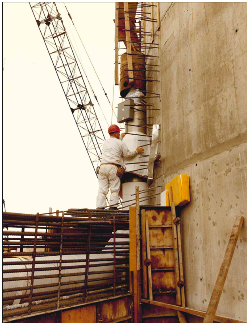
Figure 2-43. Calcined Solids Storage Facility 6 historical photograph taken during construction, showing the rebar and concrete form in place around the steel pipe in preparation for pouring the concrete encasement.
