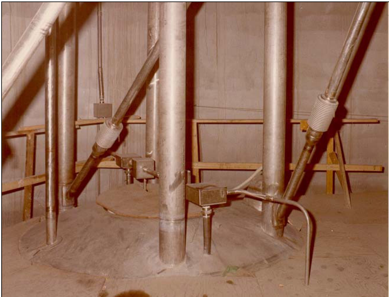
Figure 2-39. Historical photograph of the top of VES-WS5-147 in the Calcined Solids Storage Facility 5 storage vault (EDMS ID 7188224).
