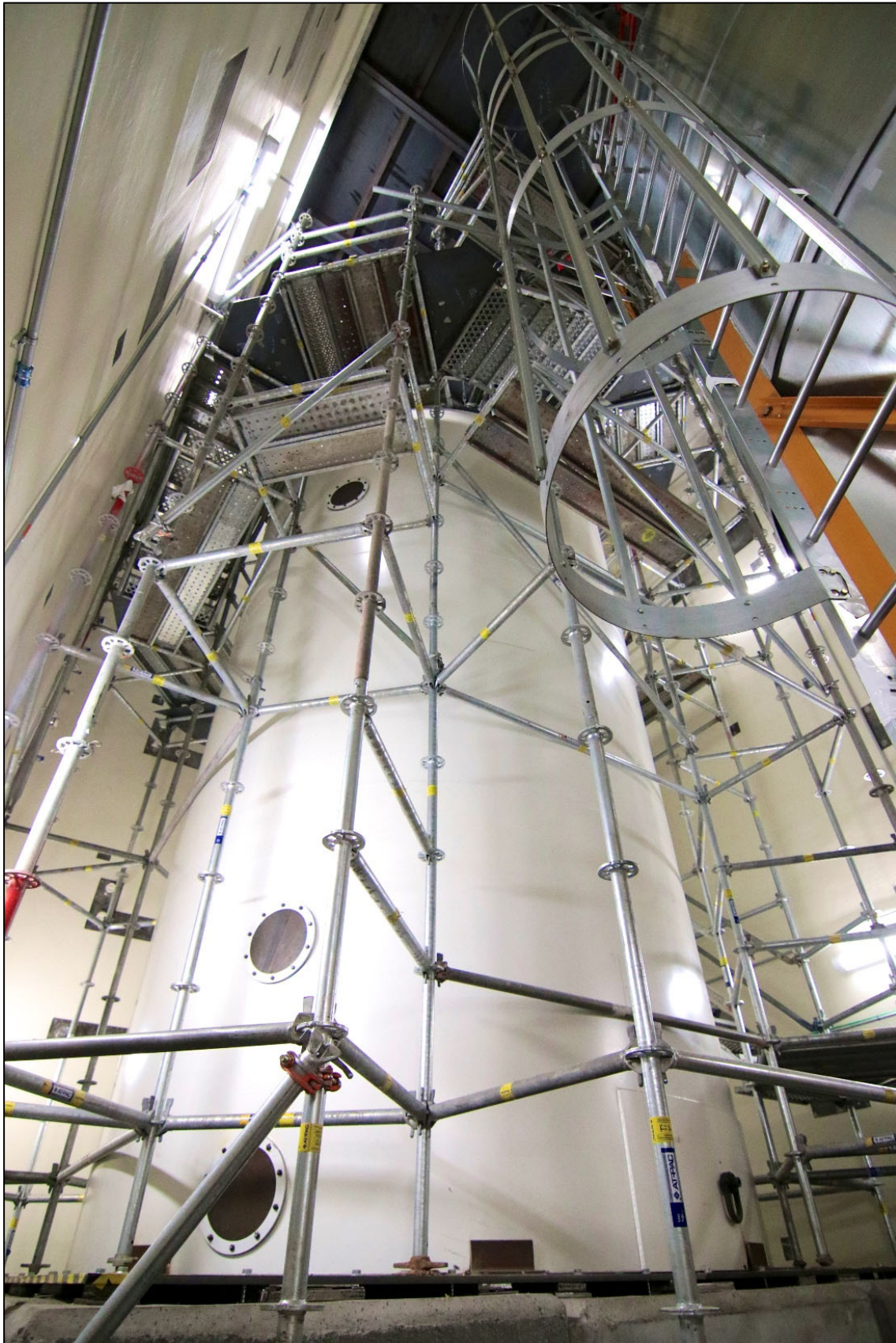
Figure 5-7. Placement of the Calcined Solids Storage Facility 1 nested bin replica in a belowgrade cell at the former Fuel Processing Restoration Facility (CPP-691).
