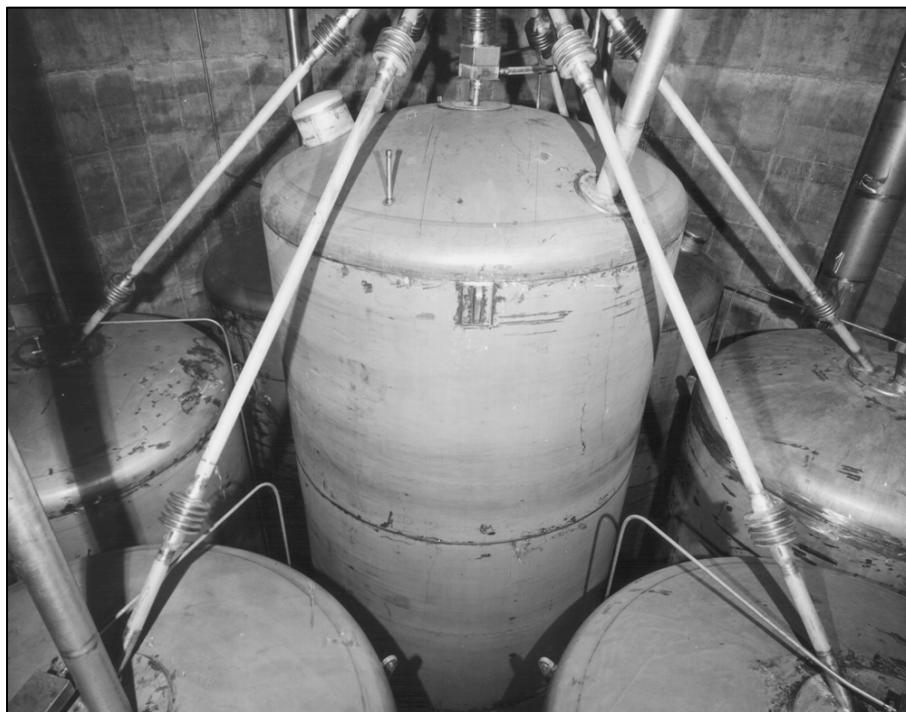
Figure 2-35. Historical photograph of center bin VES-WCS-139 surrounded by six other bins in Calcined Solids Storage Facility 3 (EDMS ID 7188225).
