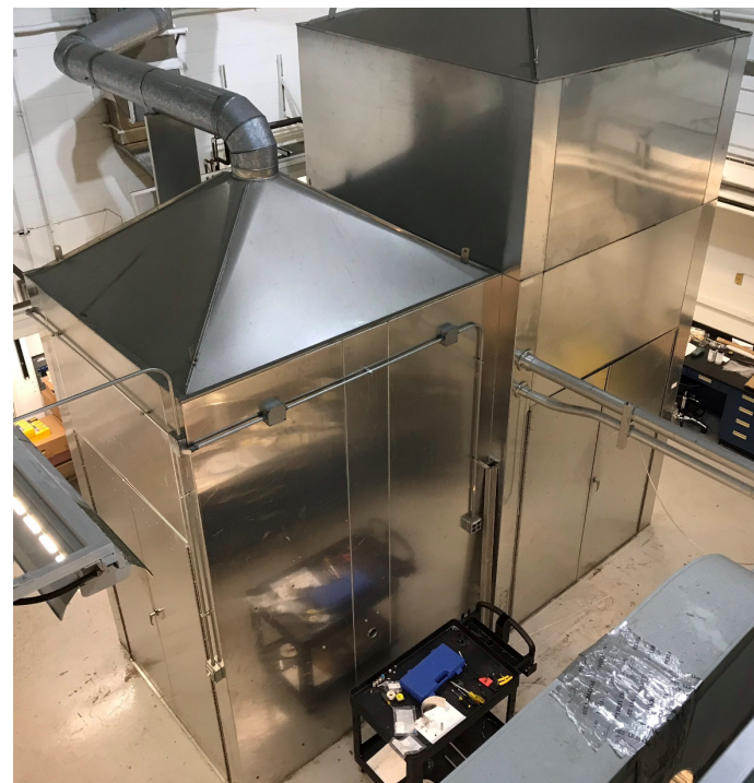
Molten salt flow loop and purification system enclosures
