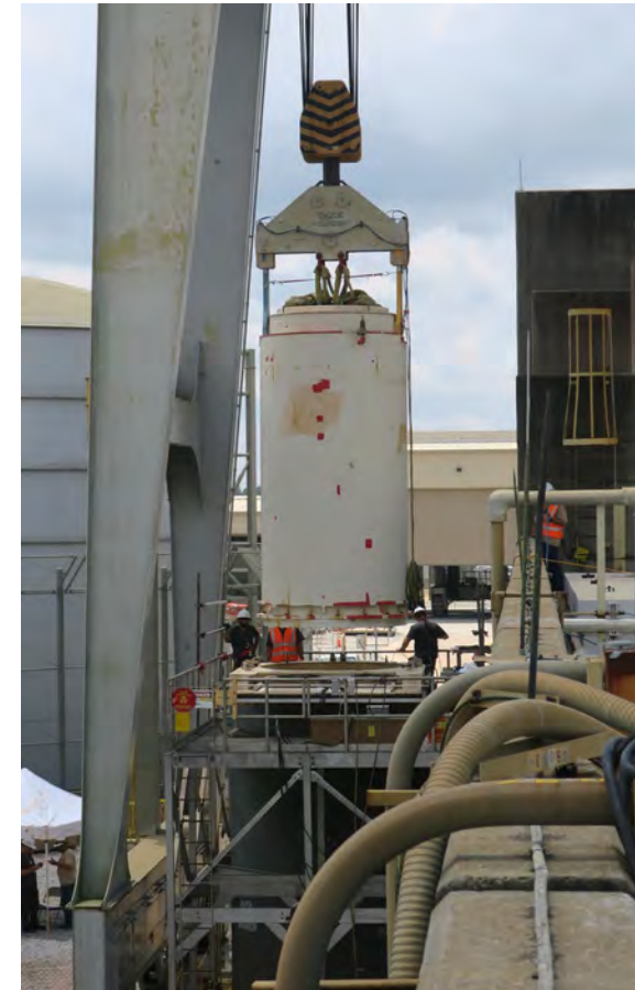
Joseph M. Farley Nuclear Plant Holtec HI-STORM 100
