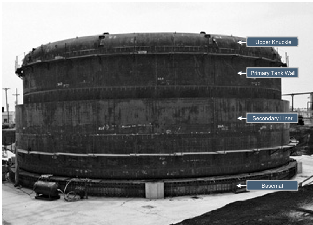
Figure 2.1-45: Typical Type IIIA Tank Primary Tank and Secondary Liner - Late Construction (Vault Wall Not Constructed)
