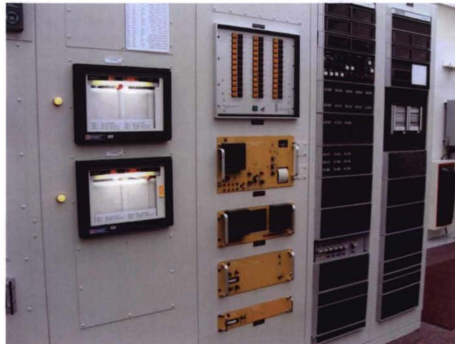
MCR Seismic Instrumentation Panel
