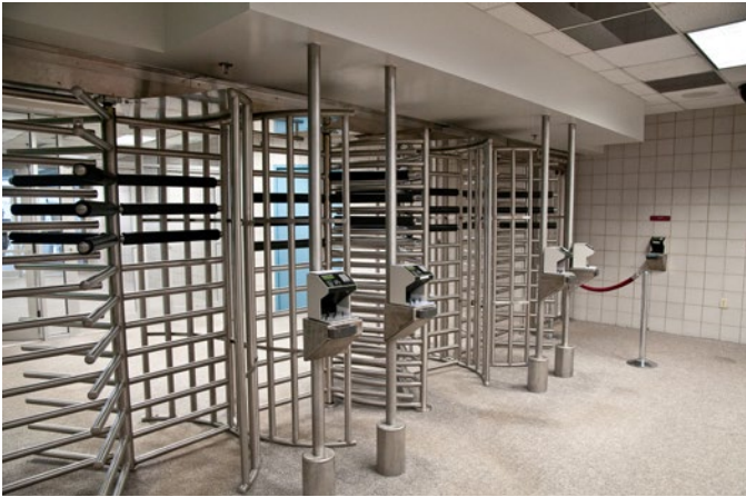
Security Access Control at a Nuclear Power Plant
